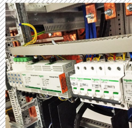
ELECTRICAL, NETWORKING, BMS & ELV SYSTEMS
